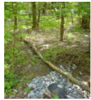
Basin at DCCD Tour Site #10
